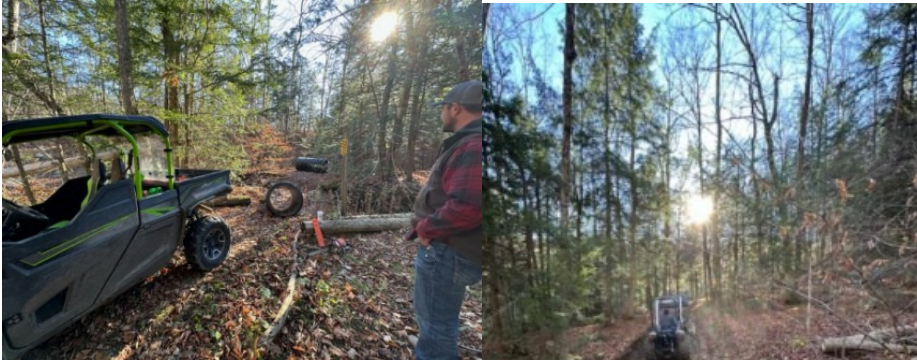
Retrieving washed out 36" culvert pipes on the S73 trail to Maple on the Lake. Photos by Trail Boss Matt Lord.
