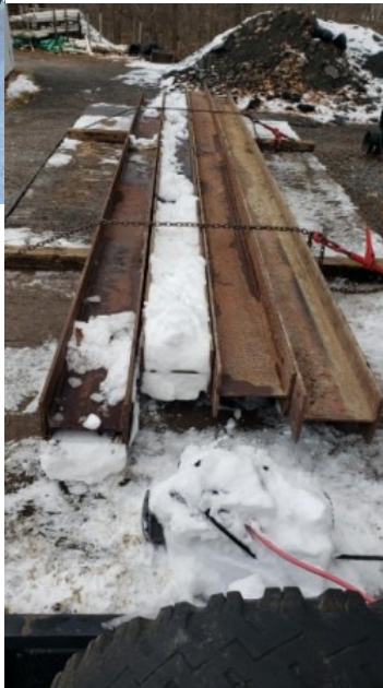
Mariaville C7B I-beams getting prepped by Justin Bates for install. Photos by Gerry Lenseth and Matt Lord.
