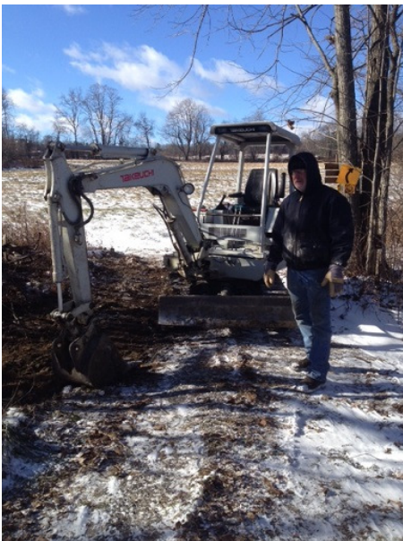
Left, Mike Wenzel looks over the culvert repair of C7B at the junction with C7G near West Road, Knox.
